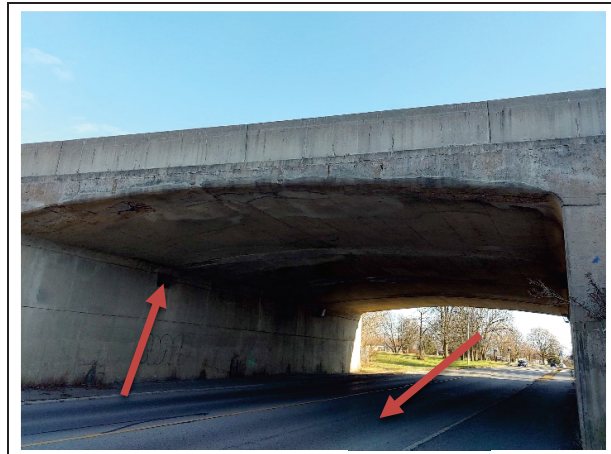
Photo 3: Lighting at Highway 401/Ormond Street Overpass (Site 16-123) suspected to contain PCB ballasts and asphalt suspected to be asbestos-containing.
