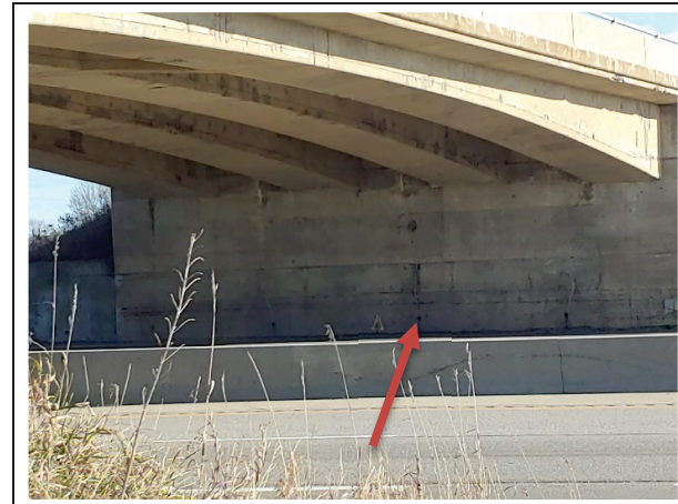
Photo 4: Presumed asbestos-containing drain pipes at Highway 401/North Augusta Road Interchange (Site 16-124).
